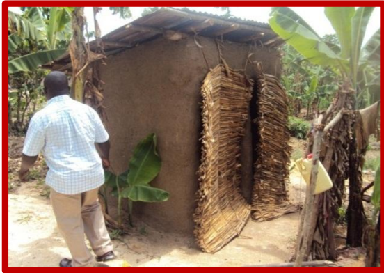
A modest pit latrine – in Nabigasa village
